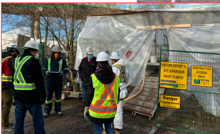
Metro Vancouver Demonstration Site
