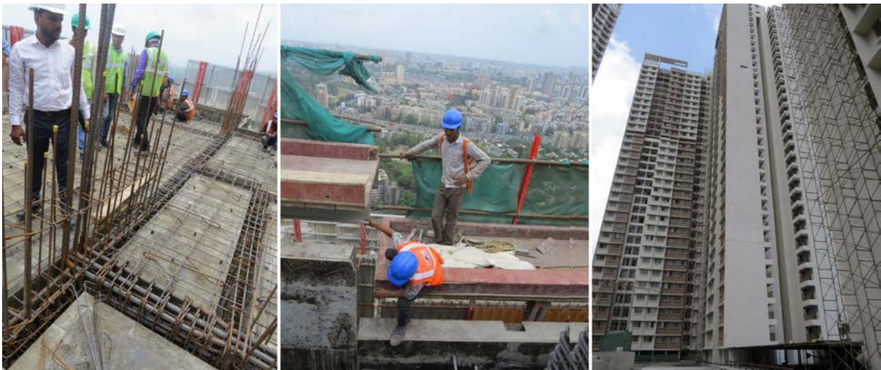
Dr. Christopoulos' team visiting construction sites and meeting with structural engineers in Mumbai
