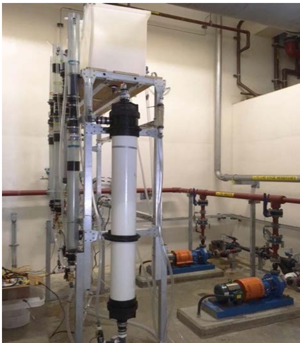
Pilot-scale passive membrane system ready for field deployment
